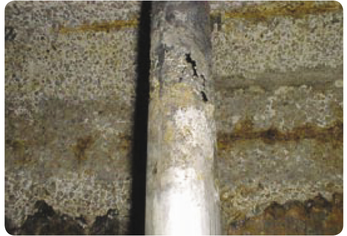
Fig. 5 Perforated Pipe Attached to the Gas Seal
