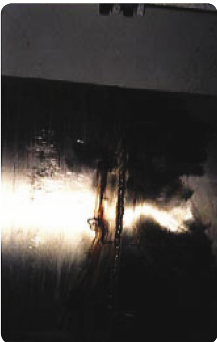
Fig. 7 Corroded Type 316 Stainless Pipe with Corrosion Product from Corrosion Attack on the Circumferential Weld.
