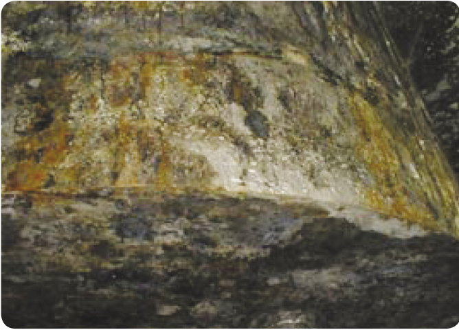
Fig. 6 Corrosion Damages on the Gas Seal
