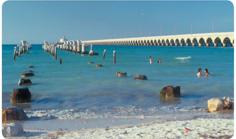
Fig. 12 Remnants of a concrete pier with mild steel rebars after 32 years (left) and a still intact pier with stainless steel rebars after 60 years (right).
